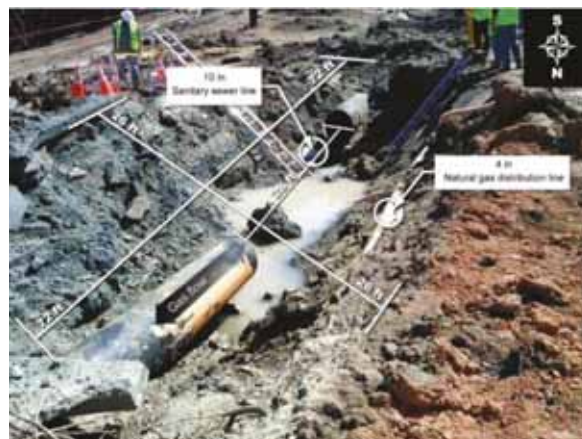
Figure 1. Pipeline Accident in California [4]
