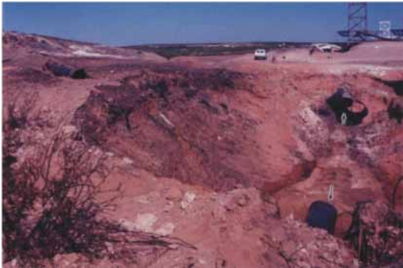
Figure 3. Pipeline Accident in New Mexico [6]
